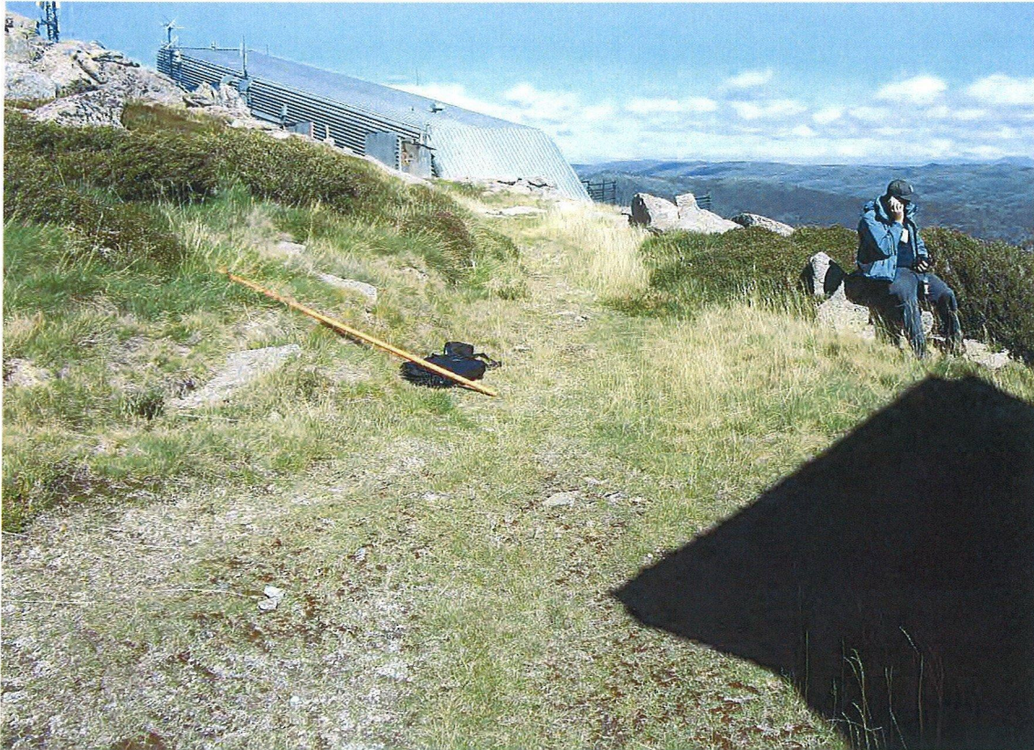
Photo 2: Disturbed area where the services trench will be located between the communications hut and the Eagles Nest building.
